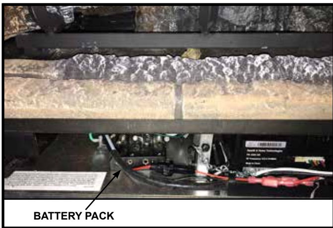
Figure 3.8 Battery Pack Installed
